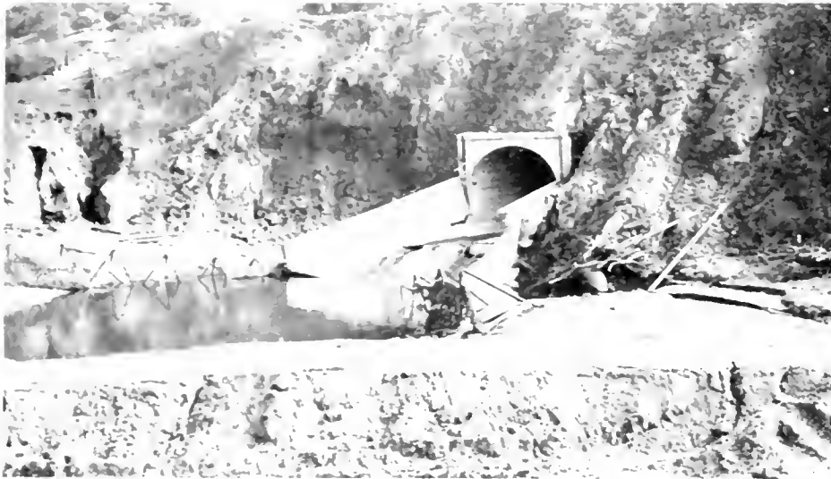
FIG. 33b. Nojoqui Creek culvert after 2000 second-foot flood of December 1941
